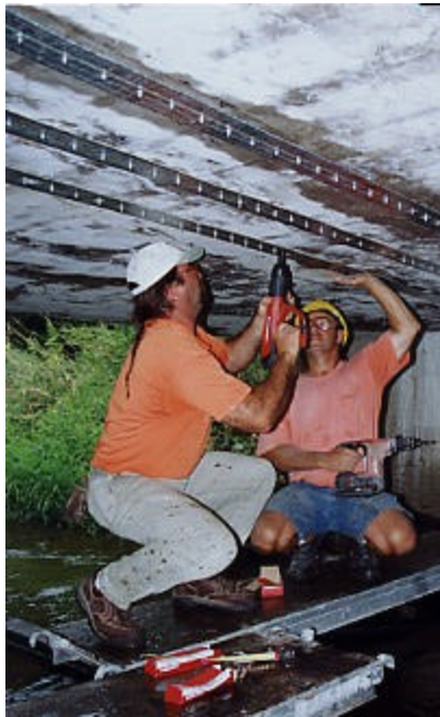
Figure 2. Installation of FRP strips on the bridge deck using Power Actuated System
